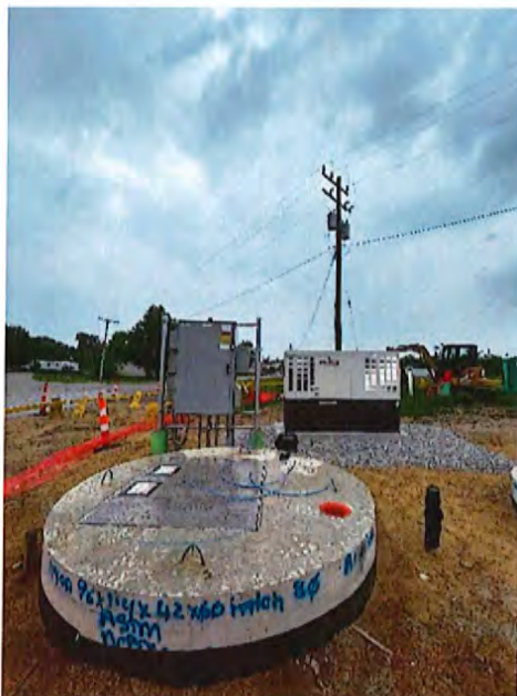
Figure 5: New Lift Station #8
