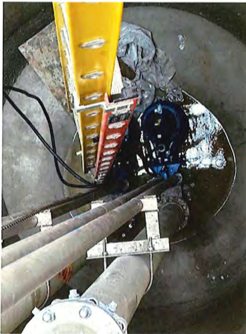
Figure 3: Lift Station #8 Pumps Installed
