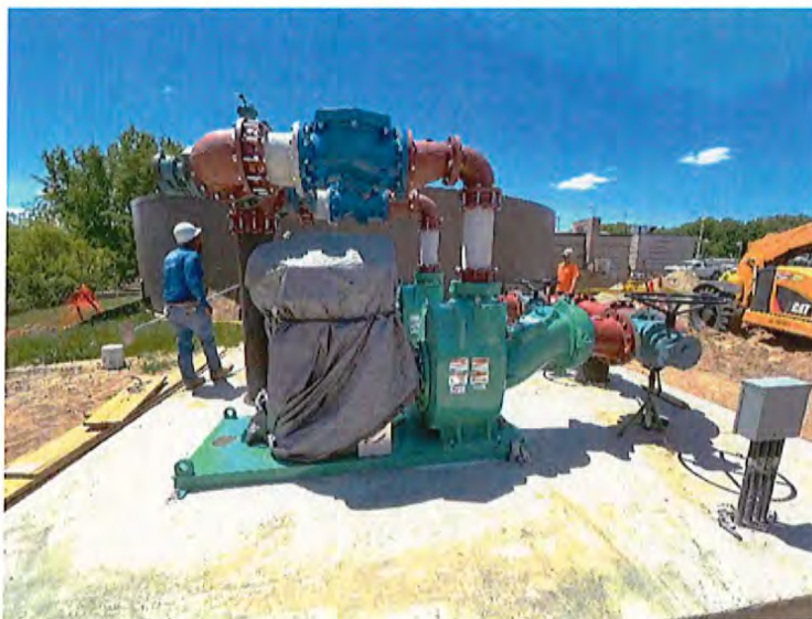
Figure 2: Digester Mixing Pumps
