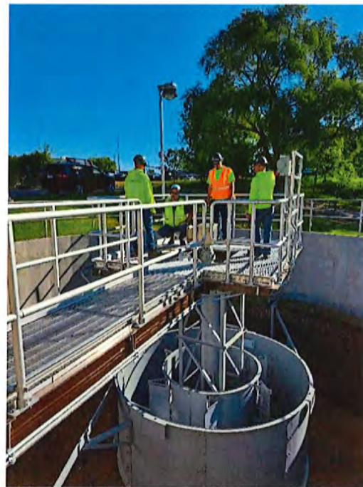
Figure 4: Manufacturer Inspecting Drives at Clarifier
